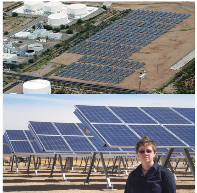
Fig. 1. The 1.6 MW system used in this study. (Top) Aerial view. (Bottom) One of the authors (A.B.) in front of the PV rows.
